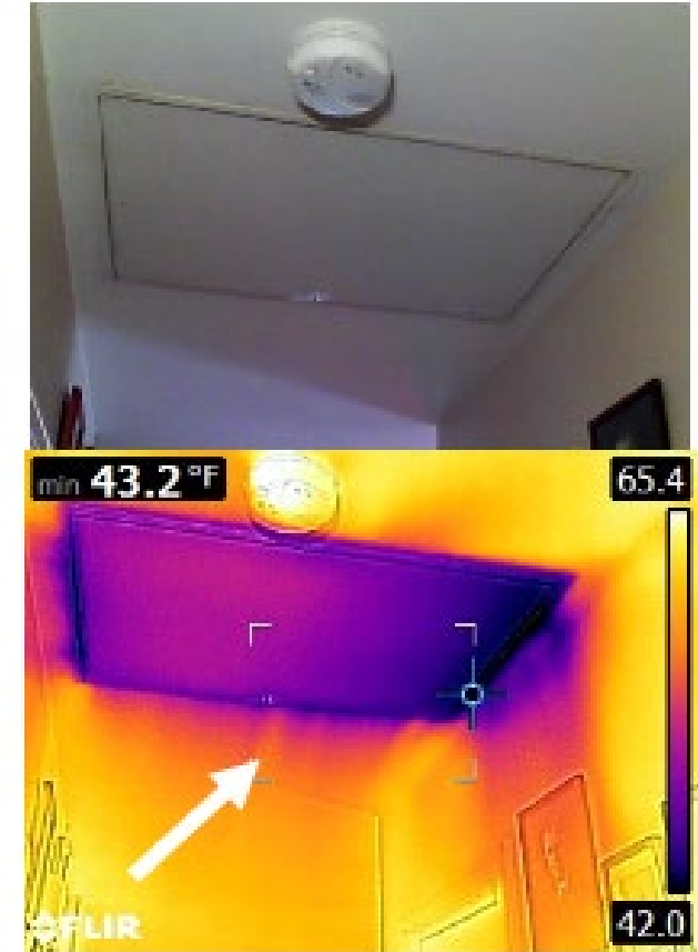
Attic Hatch without gasket
